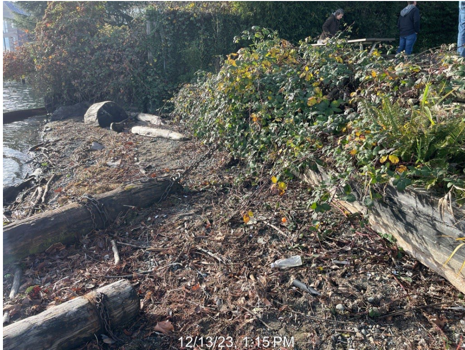
Plate 1. Looking south along shoreline of Lake Washington at failing timber bulkhead
