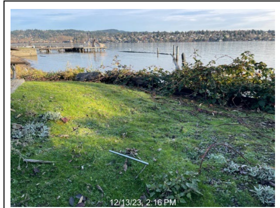
Plate 3. Note 3-foot-long steel hand probe pushed to full depth through loose fill soils.
