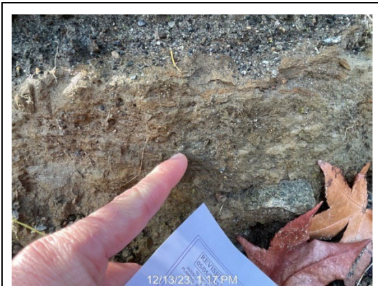
Plate 4. Exposed soils at the base of the failing bulkhead consisted of dense silty fine sand and very stiff sandy silt.
