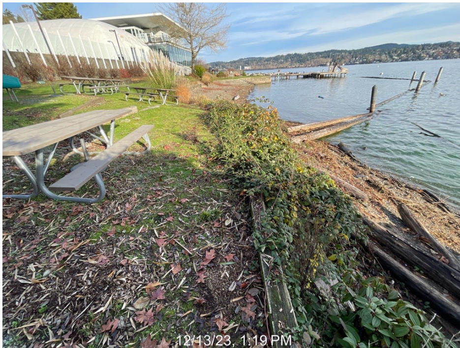
Plate 2. Looking north along top of failing timber bulkhead
